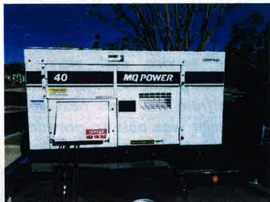
Generator supports 2-1-1VC Contact Center during Thomas Fire
